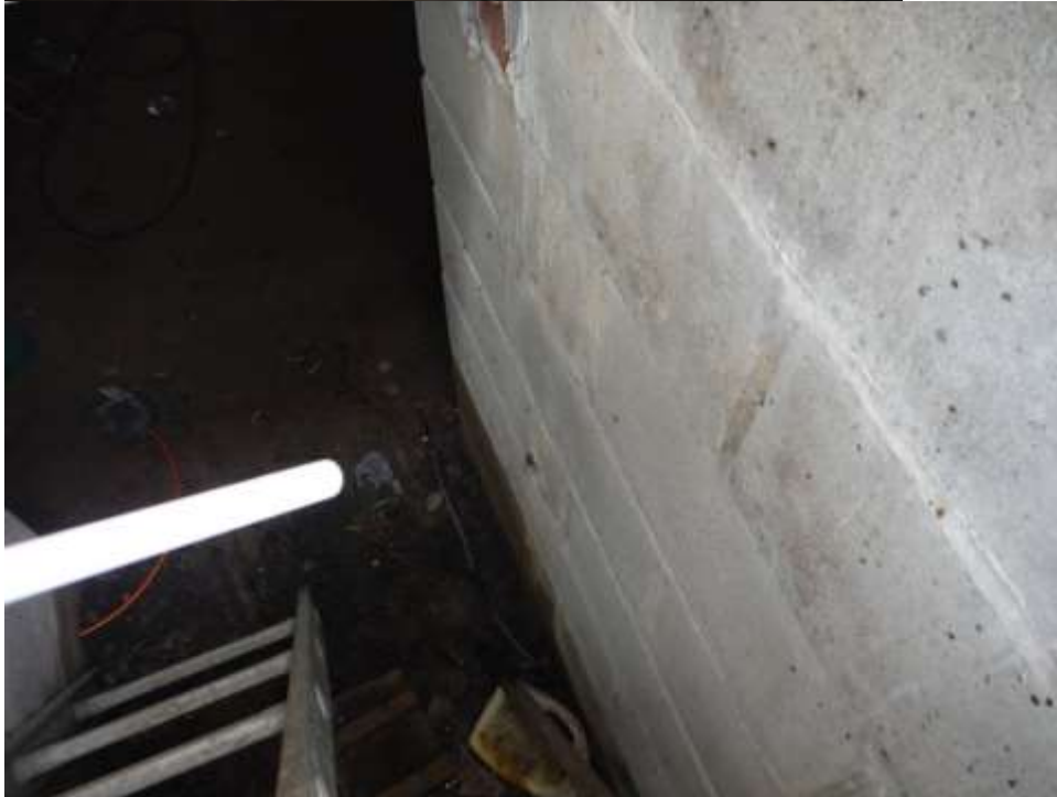
Figure 5 Example of wet conditions in the crawl space; have evaluated for grading & drainage, extend gutters, replace cover to crawl and have evaluated for encapsulation ( vapor barrier, sump pump/drains and dehumidifier).
