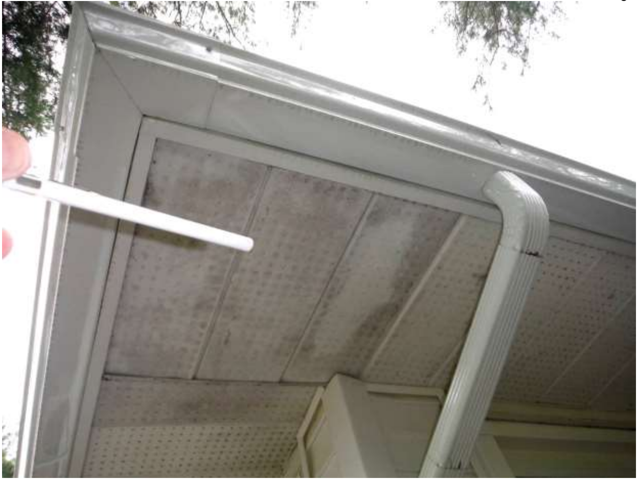
Figure 1 Example of soffits, leaking, dark staining, etc.- have evaluated by the Association before closing and all repairs where leaking & water sources into the interior.
