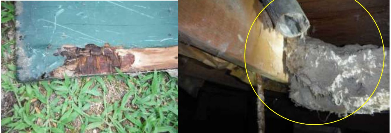
Figure 3 Rotted crawl space cover; have replaced. Example of dryer vent and lint terminating in crawl space; have vented to exterior.
