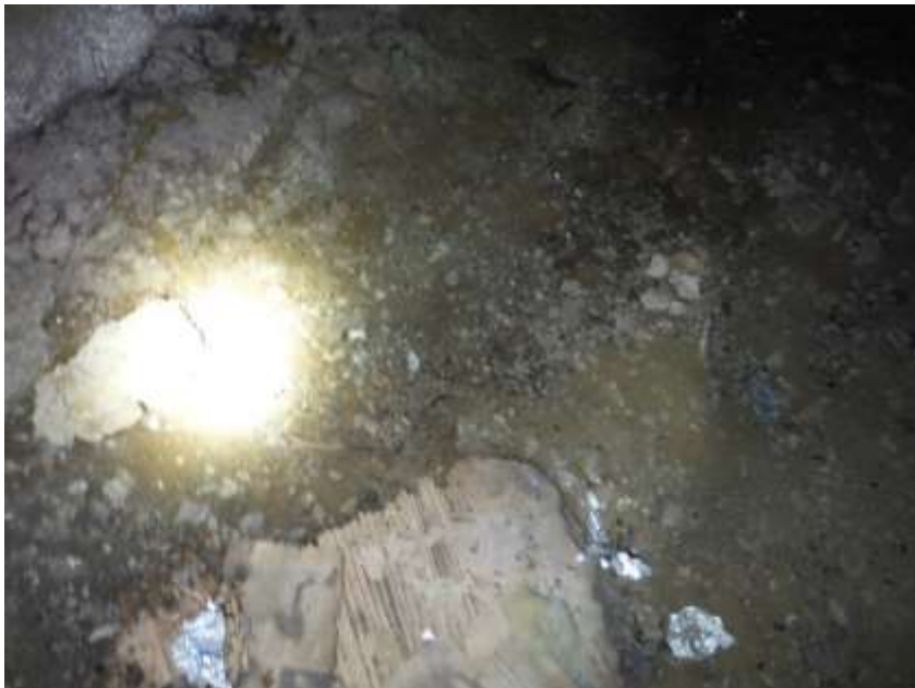
Figure 4 Puddles at opening, wet sandy soil, dryer lint, wet insulation, musty/mildew odor, etc. Recommend a wet crawl space contractor evaluate the crawl space for encapsulation, sump pump/drains and dehumidification. Recommend venting dryers to exterior (including neighbor).
