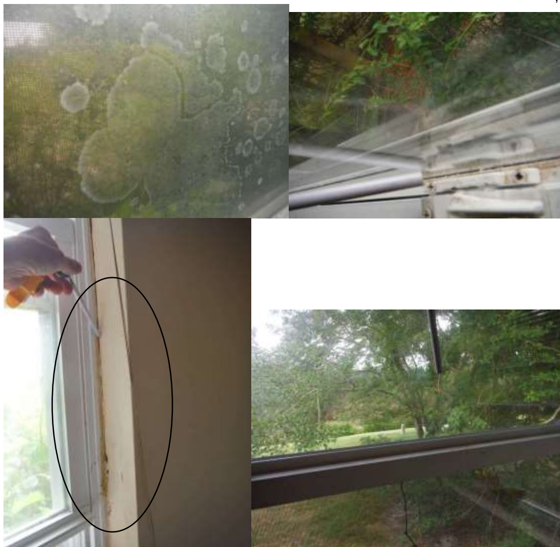
Figure 2 Example of vapor seal breaks, water damage (carpenter ants coming out of window rot), locks not aligned, window sashes not aligned, etc.
